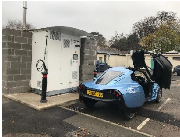
Figure 6: Abergavenny hydrogen refuelling station 30
