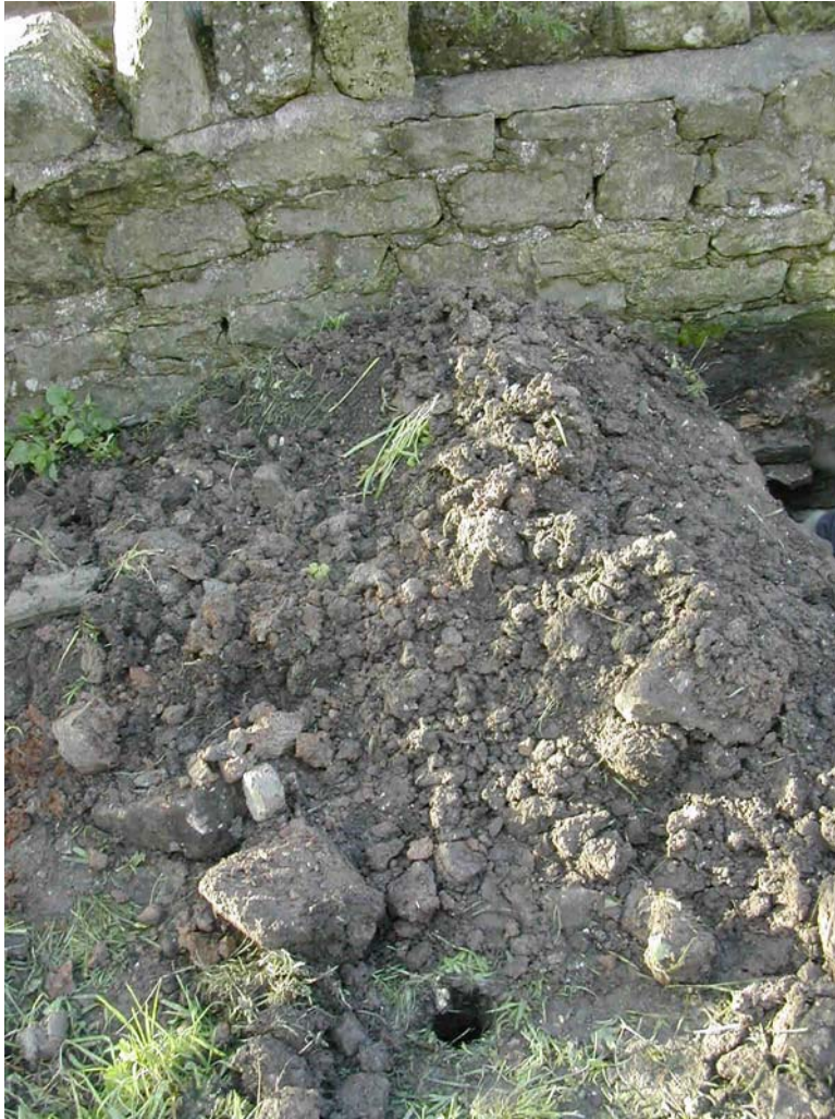
One of the bore holes in the church yard to 3.5m (approx)
