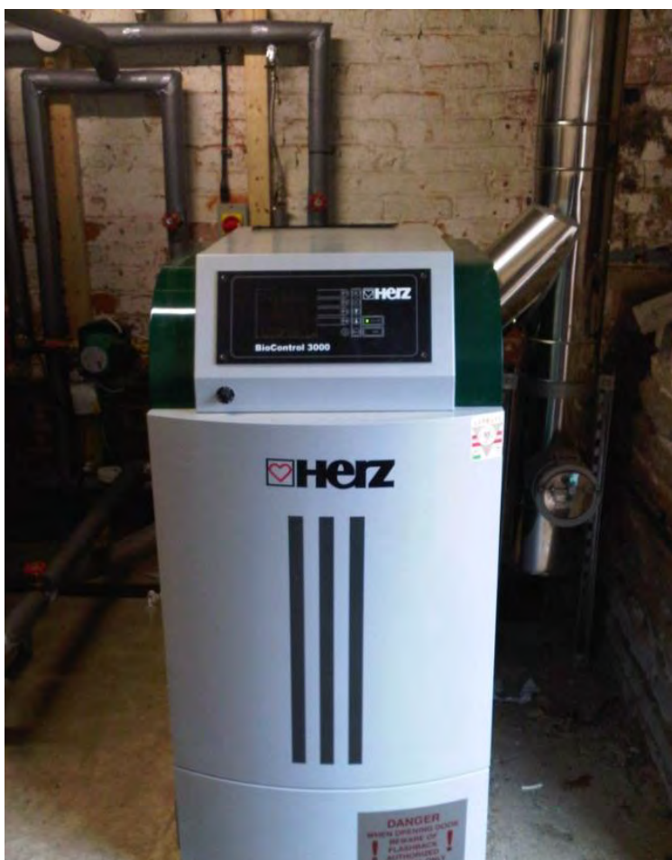
Domestic scale biomass boiler
