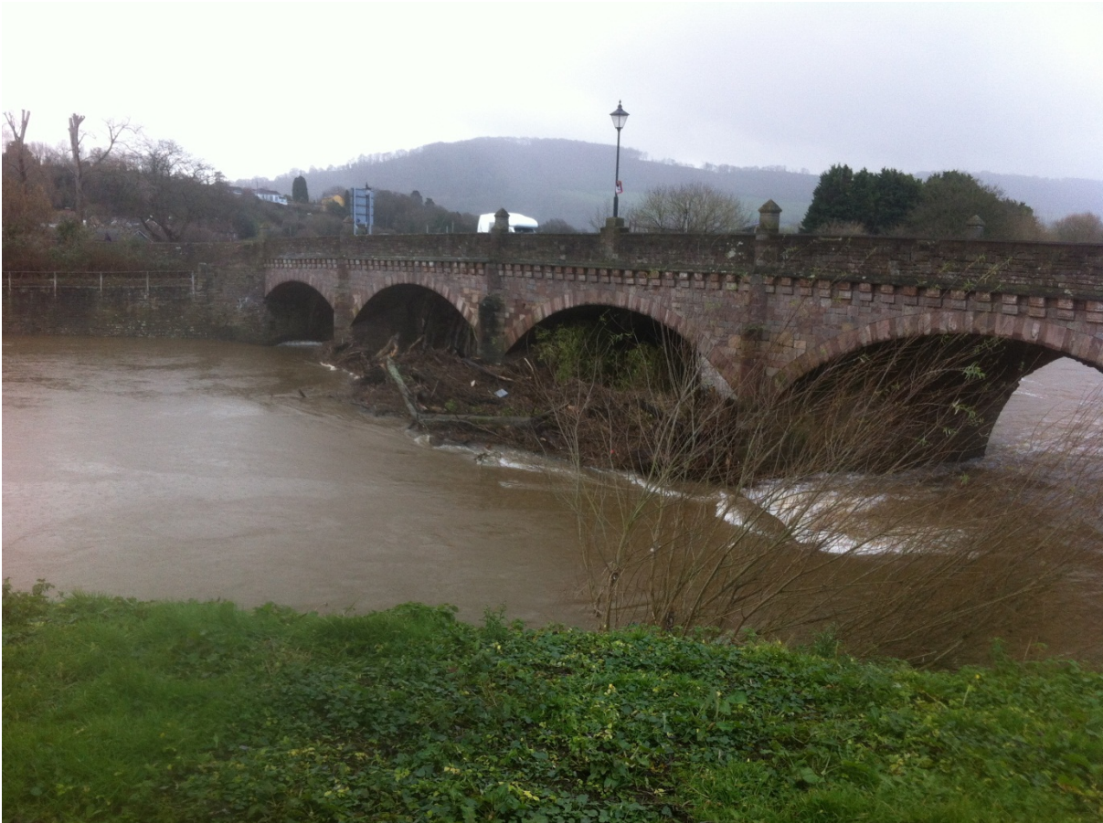
Photos of Trees & Debris Obstructing the Wye Bridge, Monmouth.
